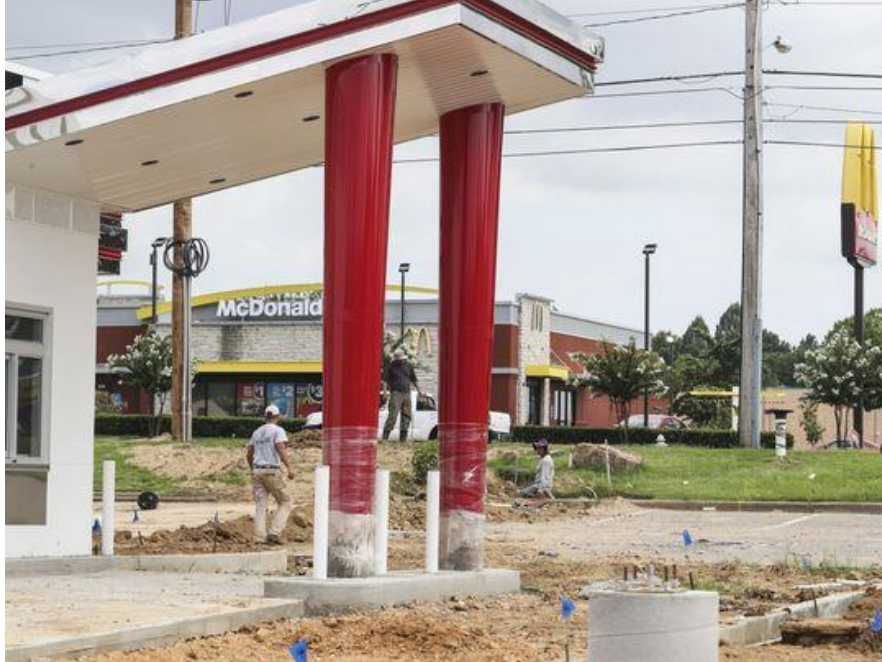
Construction continues on a new Checkers located at 6990 Shelby Drive. When it opens on July 31 it will be the 20th diner located along a 1-mile stretch of Shelby Drive. (Photo: Brad Vest/The Commercial Appeal)
