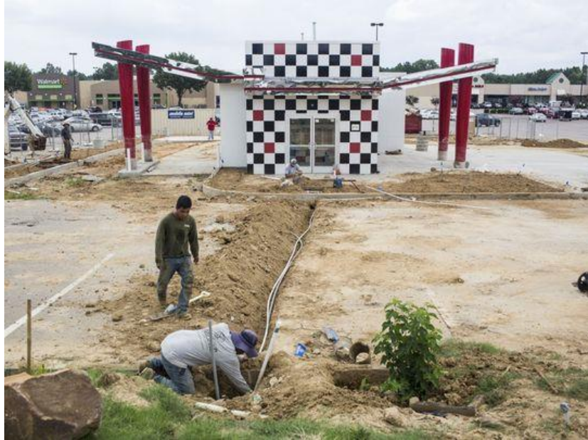
July 23, 2018 - Construction continues on a new Checkers located at 6990 Shelby Drive. When it opens on July 31 it will be the 18th fast food diner located along a 1-mile stretch of Shelby Drive. (Photo: Brad Vest/The Commercial Appeal)
